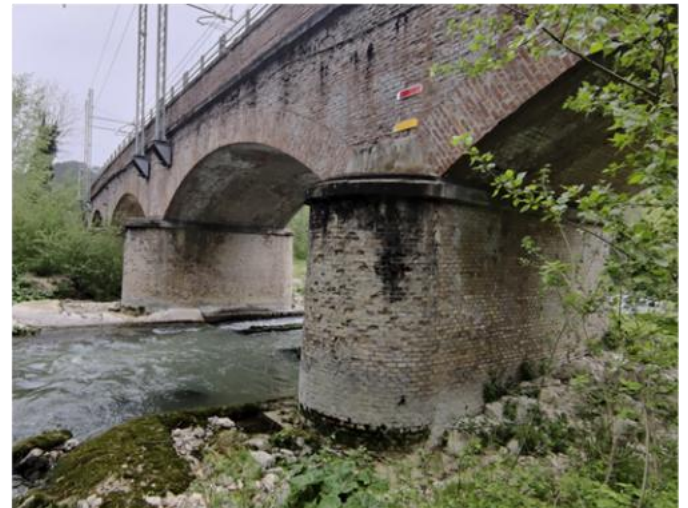
Photos of the existing railway bridge at the confluence between Sentino and Esino rivers
