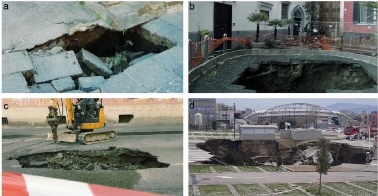
Fig. 3 Examples of sinkholes located in the city of Naples: a Via Girolamo Santacroce, Vomero municipality, 15/02/2019; b viale Calascione a Monte di Dio, 08/11/2019; c via Jacopo De Gennaro, Fuorigrotta municipality, 18/12/2019 (modified from www.ilmattino.it ); d parking of Ospedale del Mare, 08/01/2021
