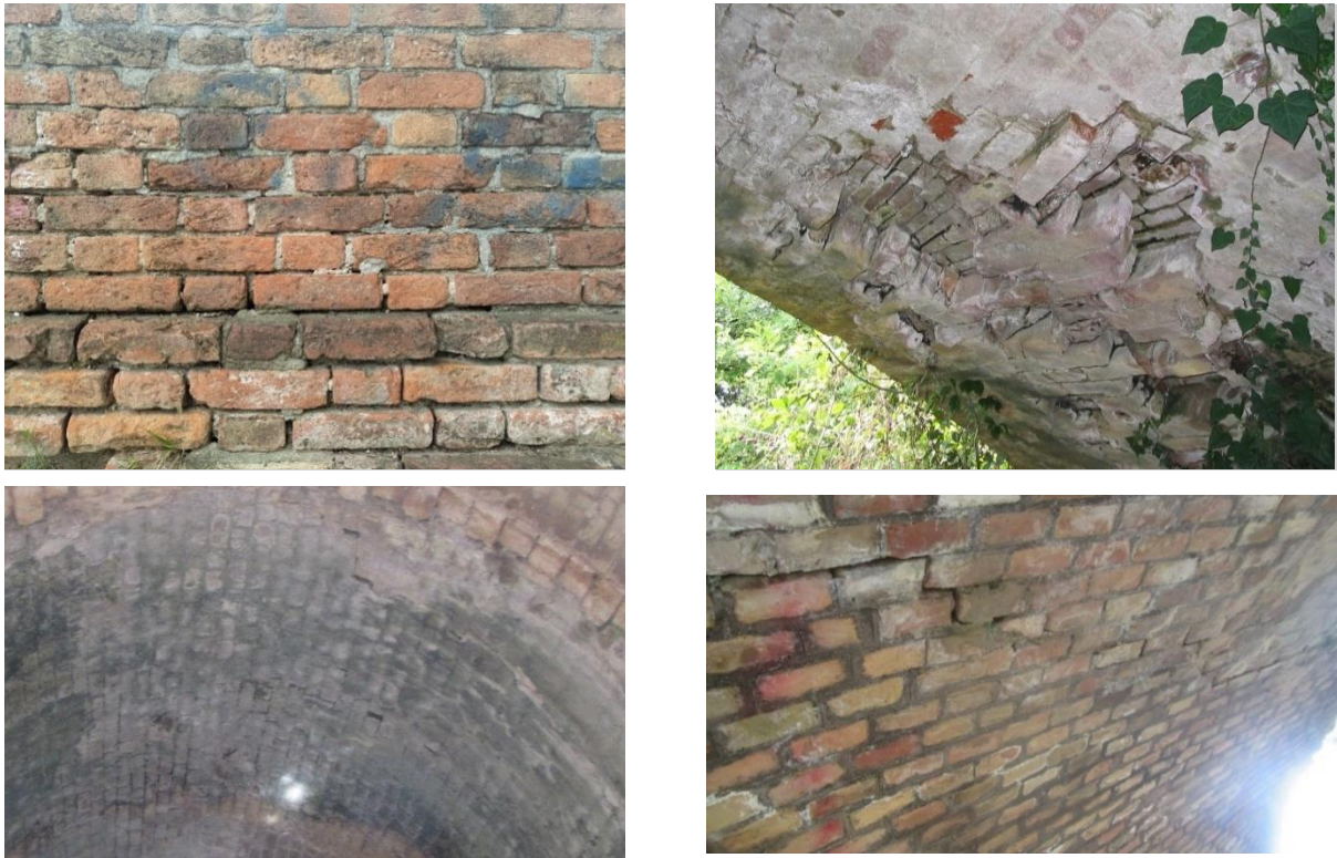
Figure 9 - Representation of some typical defect types in existing masonry bridges: (a) loss of material in the joints; (b) loss of bricks; (c) longitudinal cracking; (d) transverse cracking.
