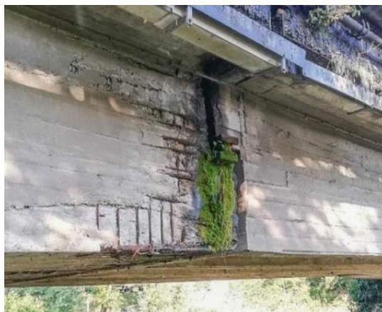
Figure 1 - Degradation phenomenon in a Gerber saddle.
